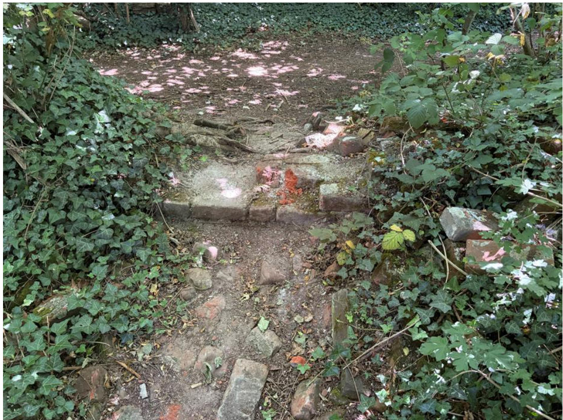
Figure 6: The West Section of the Wall has been almost entirely demolished. This includes a section that has been removed to create an informal footpath between the Warren and the Site.
