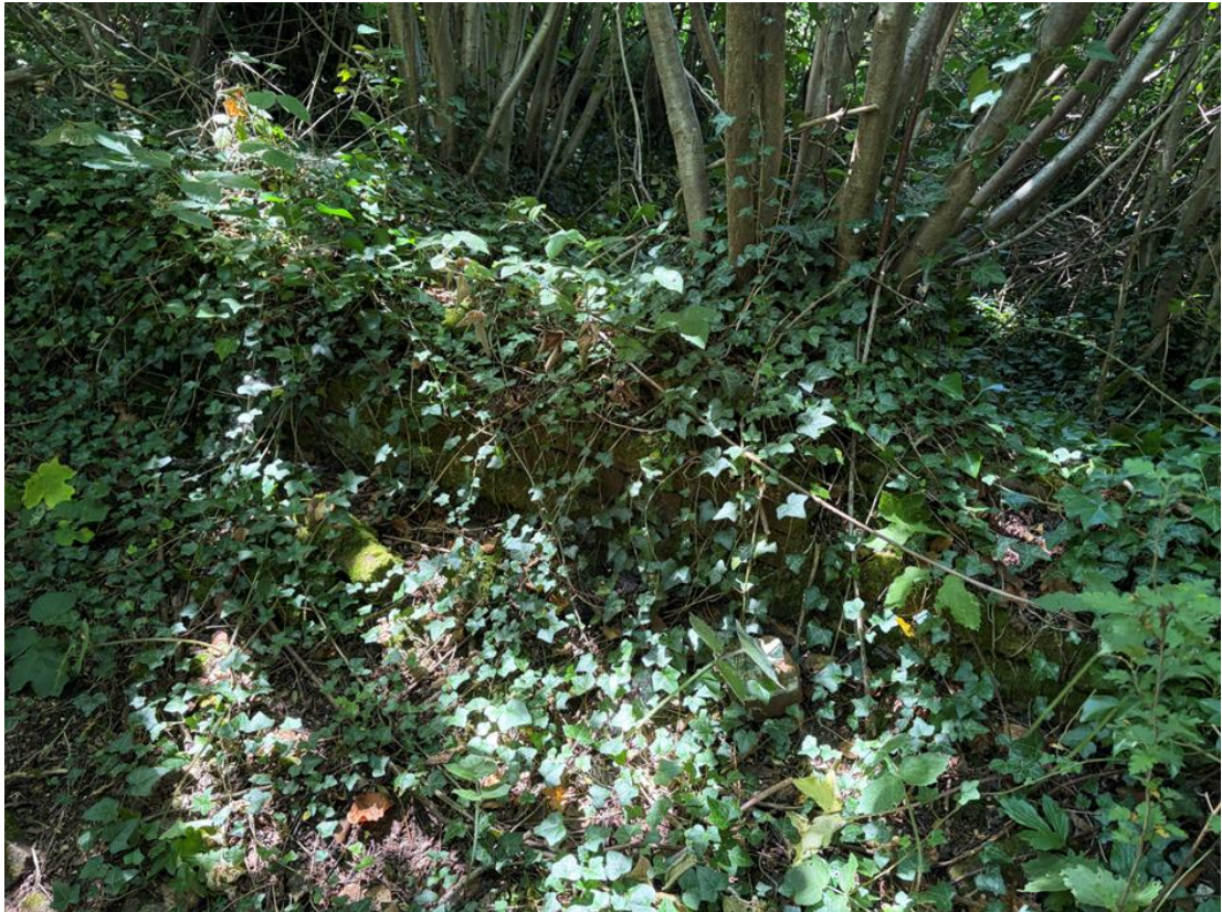
Figure 7: The Wall has suffered from vegetation growth which has damaged it and now obscures much of the structure.
